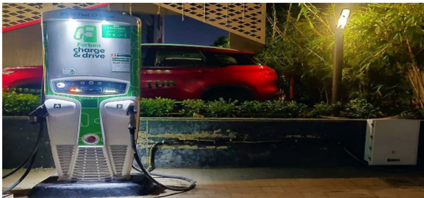
Fortum Charge & Drive India has been a forerunner and first mover in expanding the EV charging network for public charging, fleet charging, and captive e-bus and e-truck charging. Photo: Fortum Charge & Drive India
